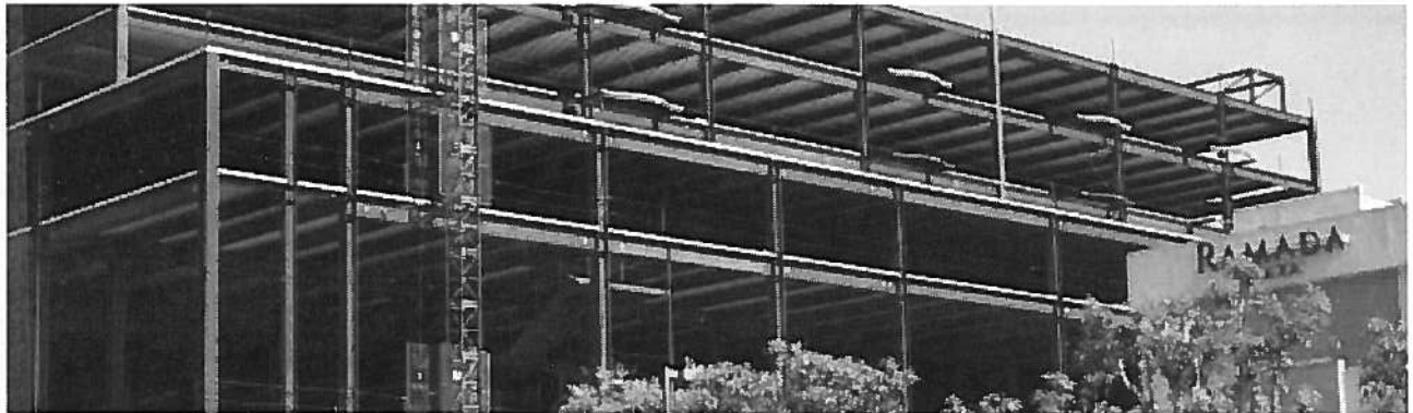
A RE-DO of what’s been called “the rusty skeleton” won approval Thursday night by Garden Grove Planning Commission on Thursday (OC Tribune photo).
