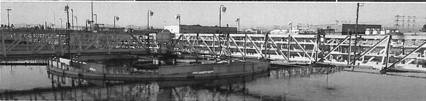
Bottom: Secondary clarifier at Plant No. 1 in Fountain Valley.
