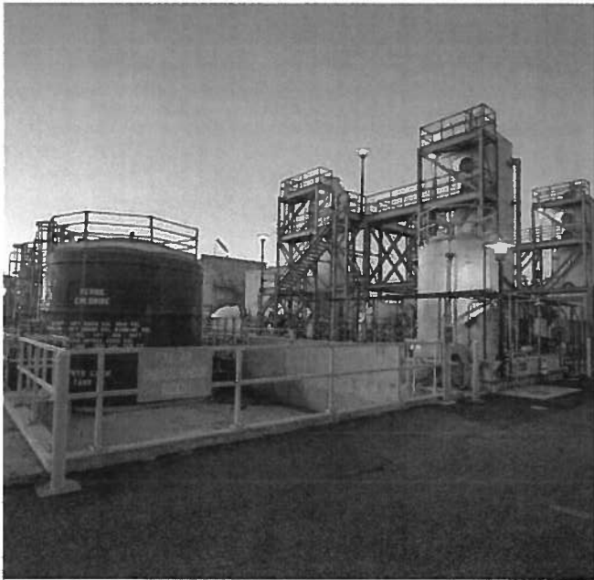
Foul air chemical facility at Plant No. 1 in Fountain Valley.
