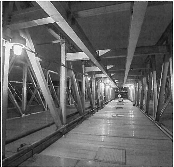
Covered primary clarifiers at Plant No. 1 in Fountain Valley.
