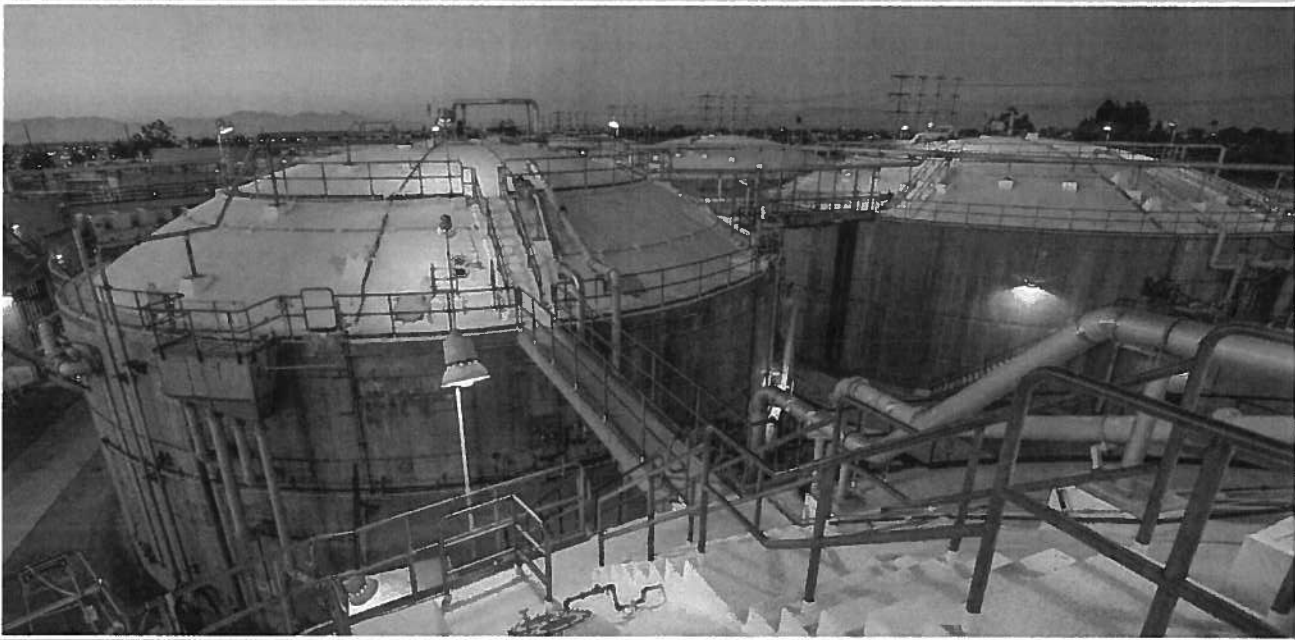
Digesters at Plant No. 1 in Fountain Valley.
