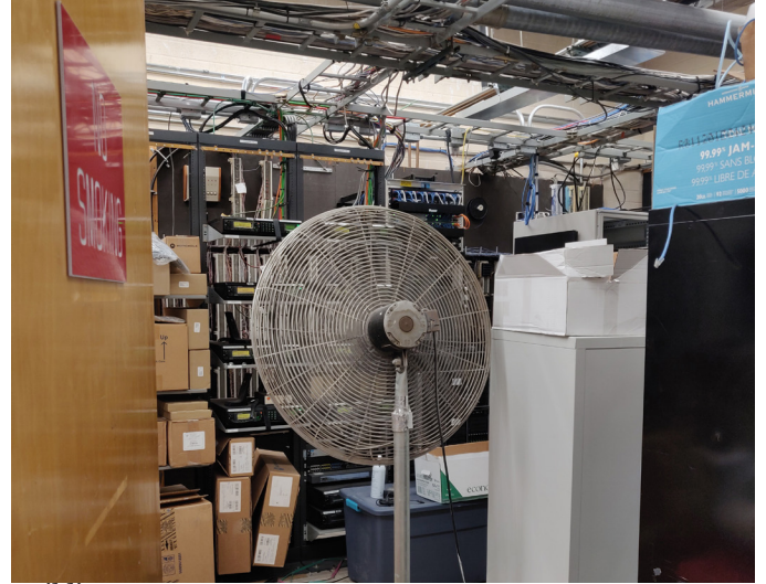
Building Server Room
